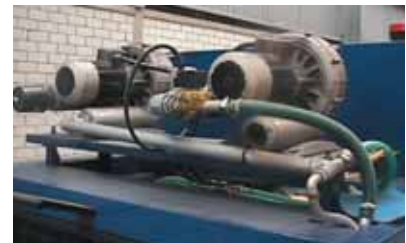
New feeder pumps
